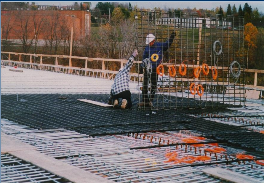
Sensors installed on FRP reinforcing grid prior to installation in a concrete bridge deck
