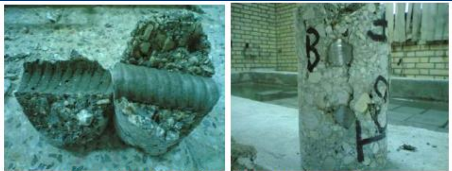
Figure . Separation of rebars after compression test of cores
