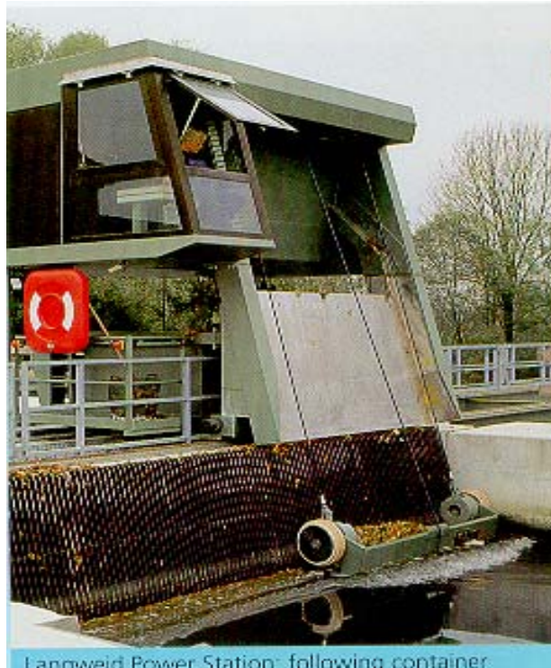
Langweid Power Station following Container
